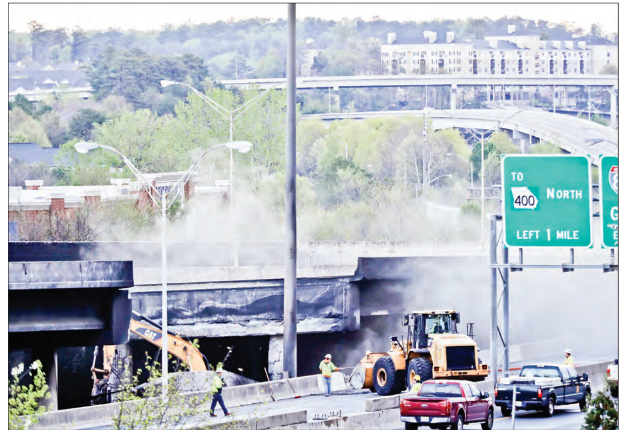
CREWS WORK on a section of an overpass that collapsed from a large fire on Interstate 85 in Atlanta, Friday. Many commuters in some of Atlanta's densely populated northern suburbs will have to find alternate routes or ride public transit for the foreseeable future after a massive fire caused a bridge on Interstate 85 to collapse Thursday, completely shutting down the heavily traveled highway.
