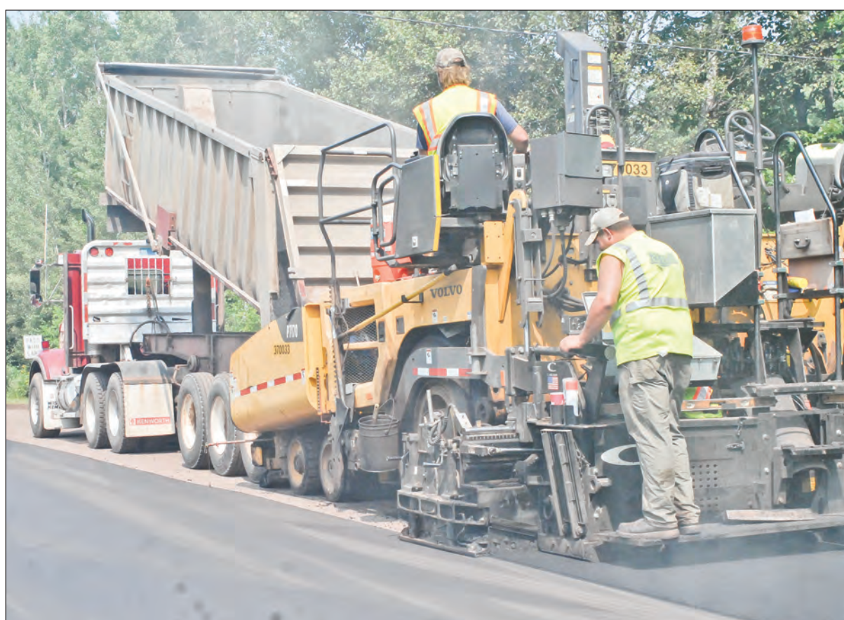
NORTHEAST ASPHALT, of Woodruff, Wis., repaves a section of Vanderhagen Road in Ironwood Township Thursday. Among those working on the road are, from left, Tim Kiel and Andrew Burzynski.
